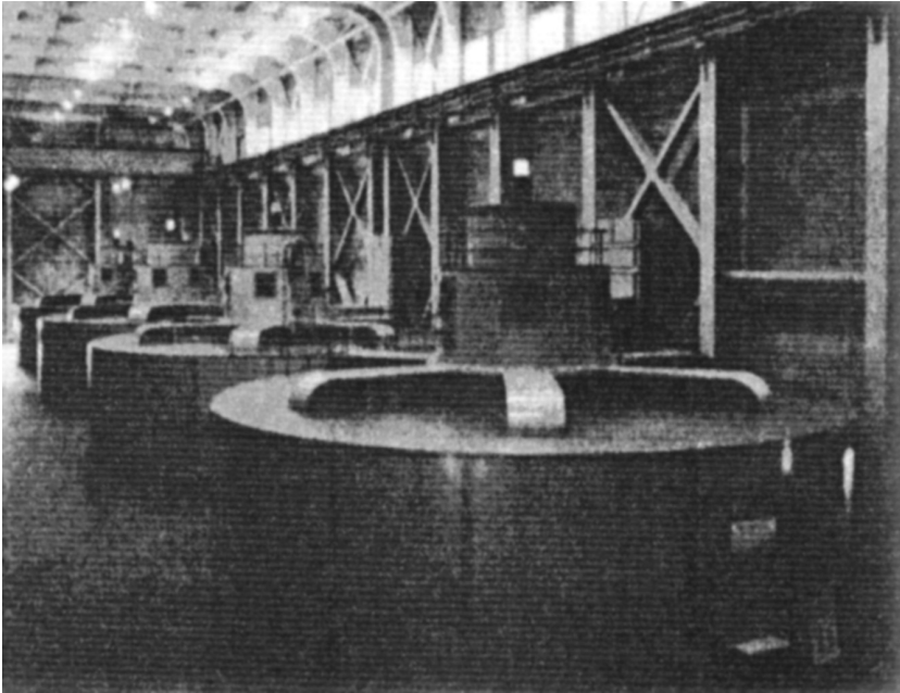
FIGURE 8.1 Four 100 MVA, 13.8 kV vertical-shaft hydrogenerators. The hydraulic turbines (not shown) are located on the floor below. (Courtesy of Seattle City Light.)
