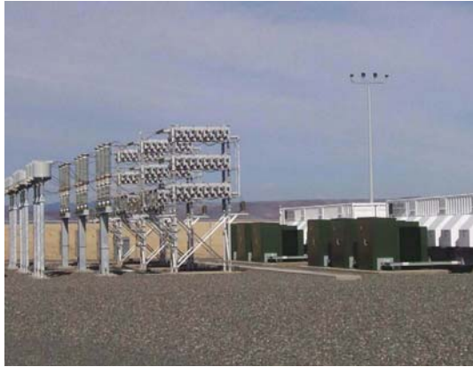
Figure 15.13 Reactive compensation system rated +78/−12 MVAR including three stages of switched capacitors, 22 MVAR each, and dynamic capability of ±12 MVAR continuous and ±33 MVAR short time (Courtesy of S&C Electric Company)
