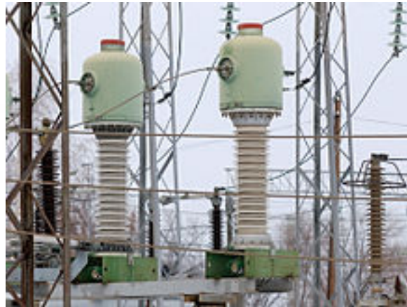
SF6 110 kV current transformer
