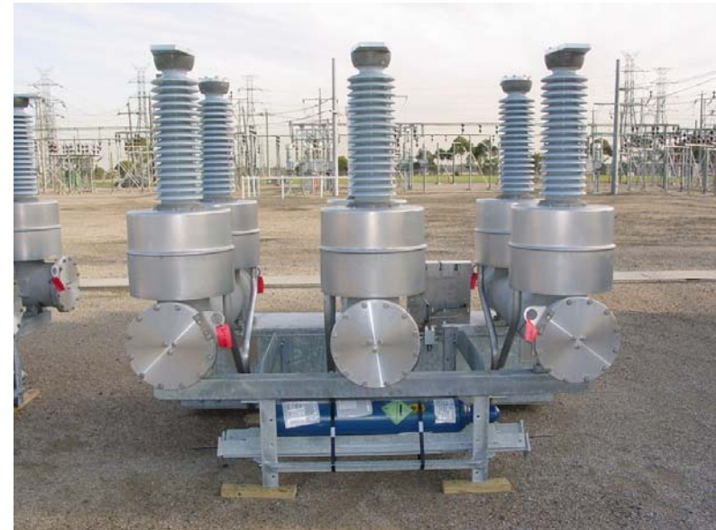
Bushing-type CTs installed on the bushings of 66kV Dead Tank Breaker
